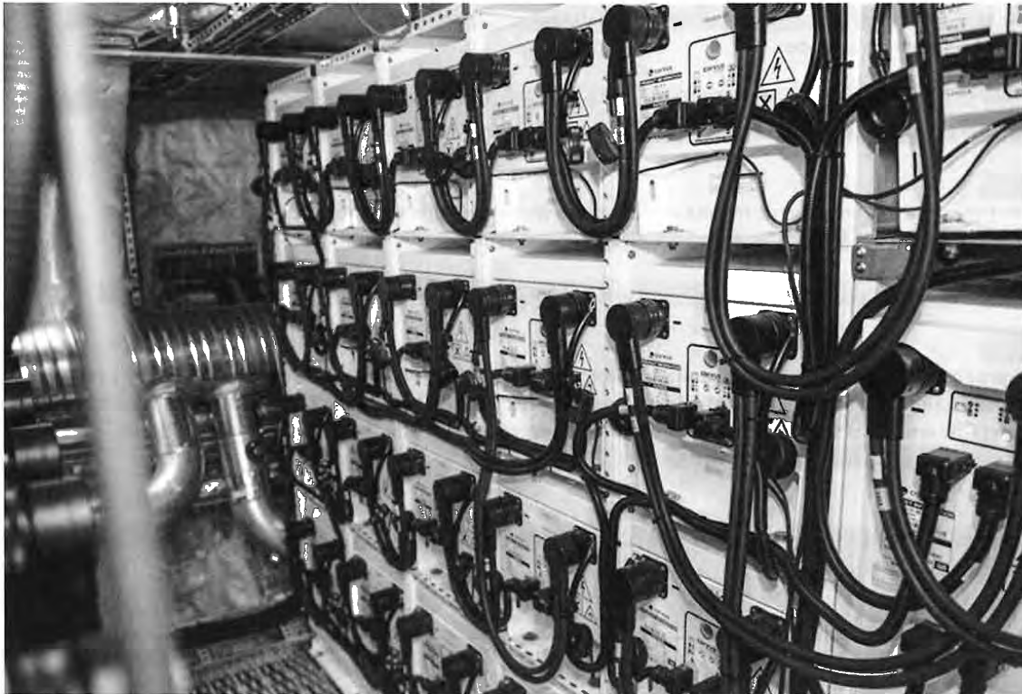
Cables connect to batteries in the battery room of the MF Ampere.
