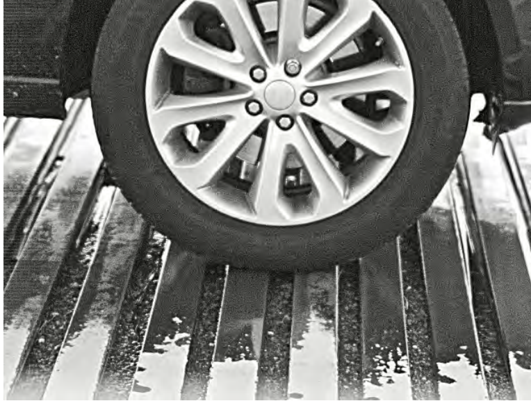
Figure 5-18 Frame from high-speed video recording of an SUV tire passing over east-side large expansion joint center beams.
