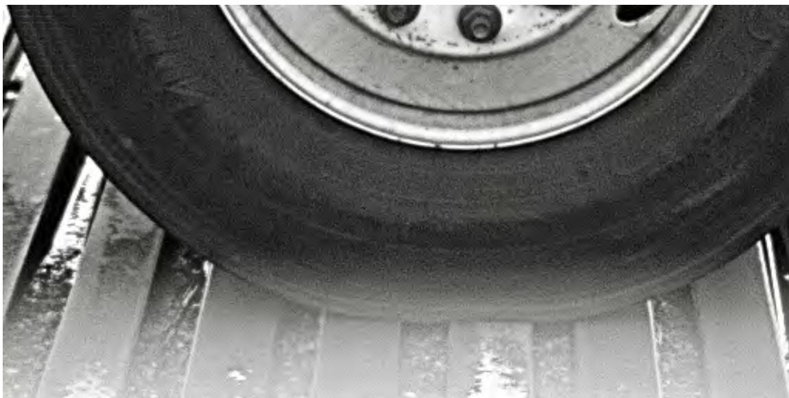
Figure 5-21 Frame from high-speed video recording of a bus front tire passing over east-side large expansion joint center beams.
