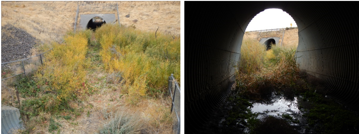
Figure 8. Historic livestock management culvert below I-90; elk were unwilling to use this potential crossing due to its small and confining nature.
