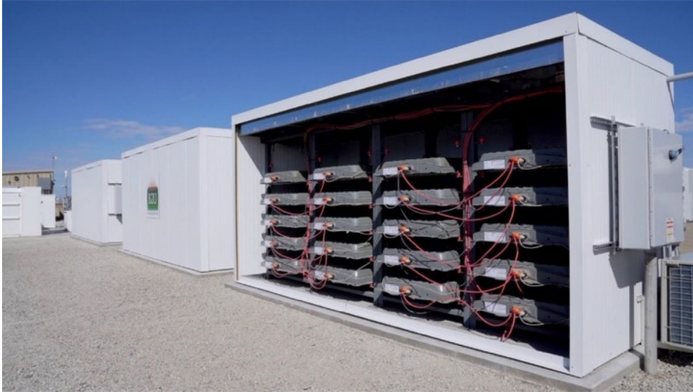
Figure 4. B2U’s UL certified EV Pack Storage (EPS) System enables the use of EV battery packs without reconfiguration in large scale energy storage 17 .
