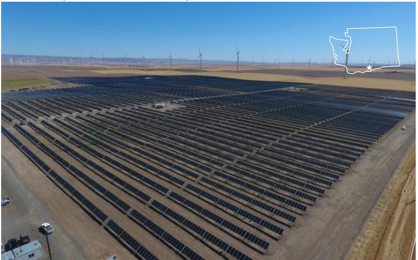
Photo: Courtesy of Iberdrola Group
