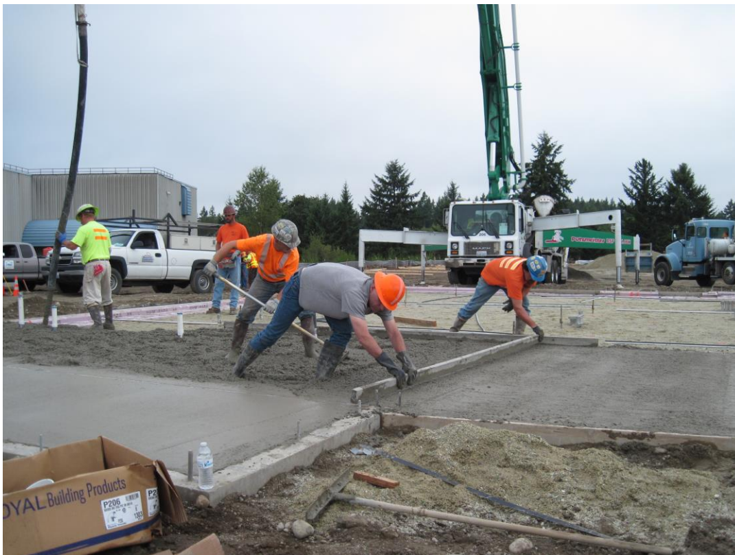
As the foundation of the community building was being poured, Rep. Timm Ormsby (in grey shirt) stepped in to help.
