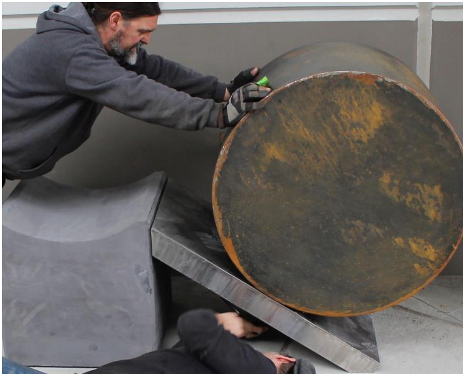
Bruce Anderson and an assistant installing Bruce and Shannon Anderson’s sculpture, Inclined Plane , part of the series Simple Machines (2016) for Green River College, in Auburn.
