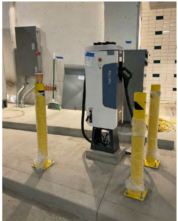
In-the-field opportunity charging at Commerce Street transit center.
