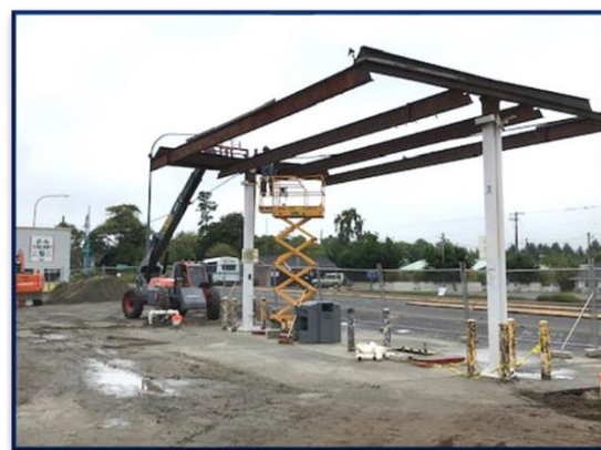
Cleanup and construction included removal of the canopy and dispensers to access tanks.
