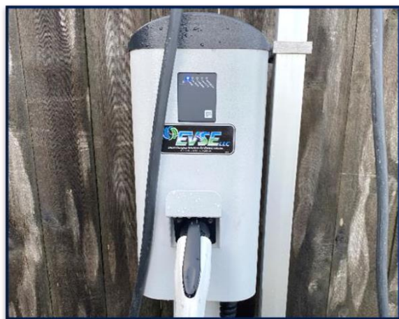
New electric vehicle charging station installed.
