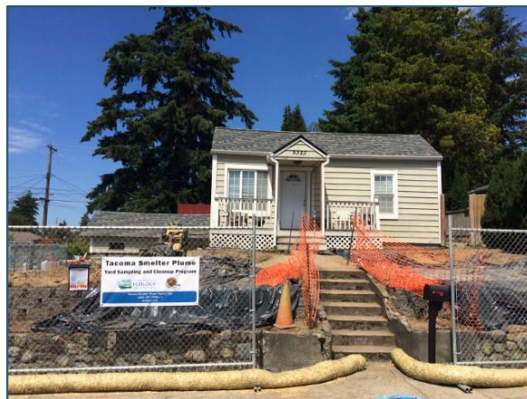
Photo 3: Contractors removed the top 18 inches of contaminated soil at a home in Tacoma.
