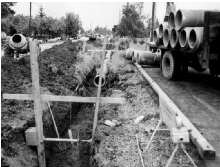
NW 78th St Pipeline Installation, 1960, Unknown, Clark County Public Works, Road Construction Photographs, 1949-1961, Washington State Archives, Digital Archives, http://www.digitalarchives.wa.gov , October 17, 2010.
