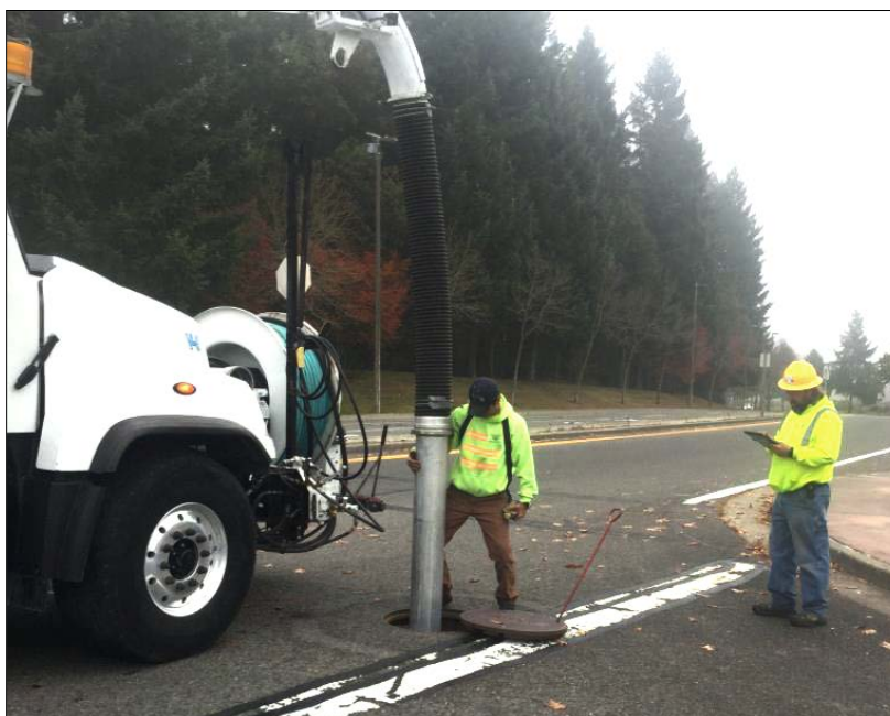
Figure 34: City of DuPont staff clean and monitor catch basins using new tracking software. Photo credit: Washington State Department of Ecology
