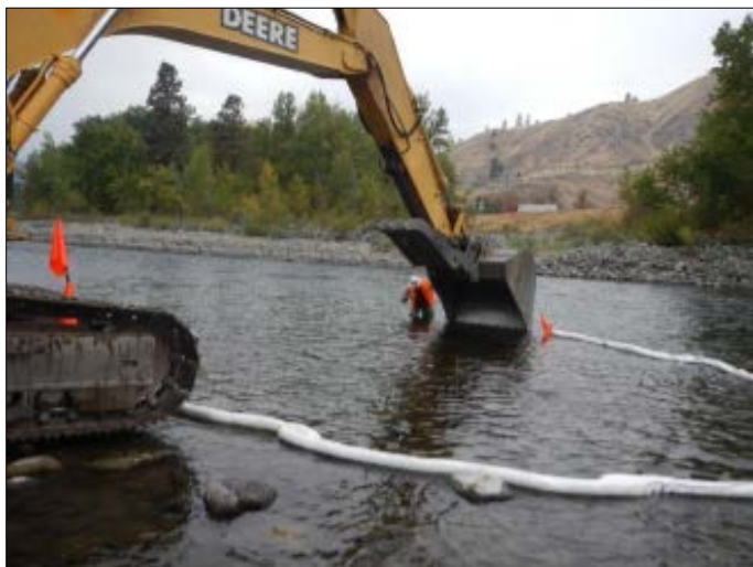
Figure 38: Removing a waste transformer in the Wenatchee River in Central Washington. Photo credit: Washington State Department of Ecology
