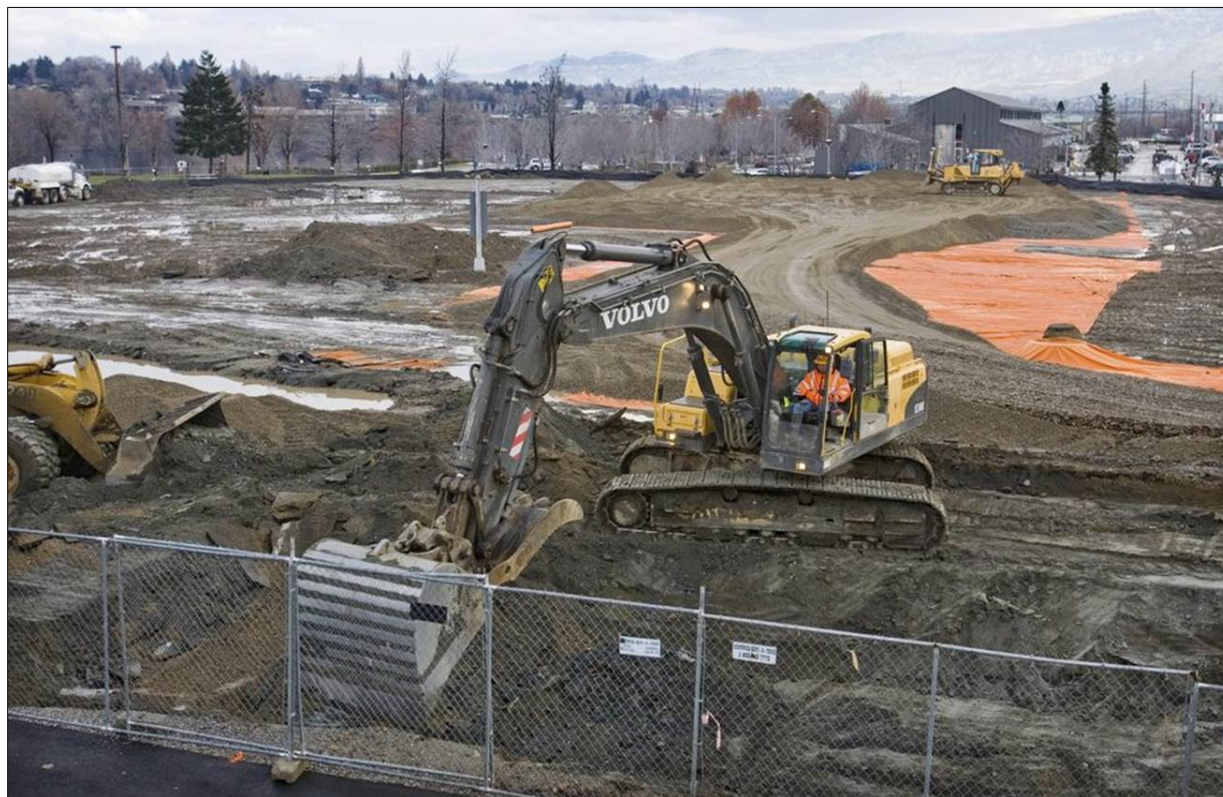
Figure 37: Before construction could begin on the new Wenatchee hotel, cleanup contractors removed contaminated soil from the site, then capped it with a foundation of the new building footprint, parking lot, and landscaping. An Environmental Covenant was recorded for the property to ensure the cap remains in place. Photo credit: Washington State Department of Ecology, 2015.
