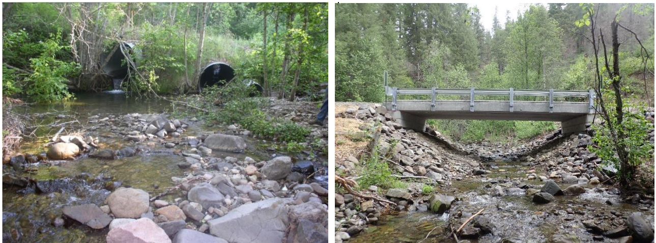
Culvert replacement with a bridge on North Nanamkin Creek on the Colville Reservation. Photo by Confederated Tribes of the Colville Reservation.
