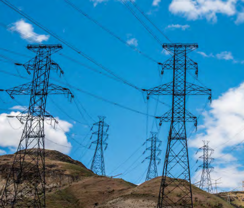
Hydroelectric power plant and transmission at the Grand Coulee Dam, WA.
