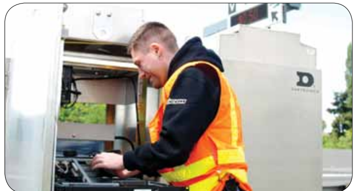
WSDOT HOT lanes technician Allen Mushatt checks the electronic equipment cabinet.
