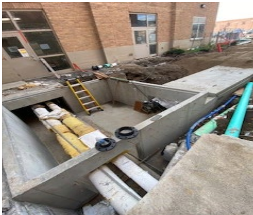
Steam and condensate return lines
