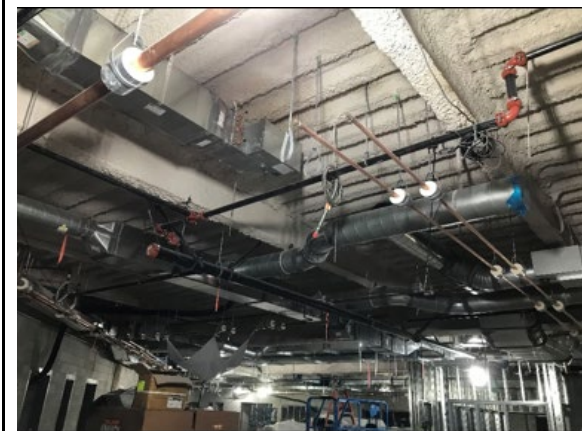
HVAC ductwork, fire sprinklers, and plumbing
