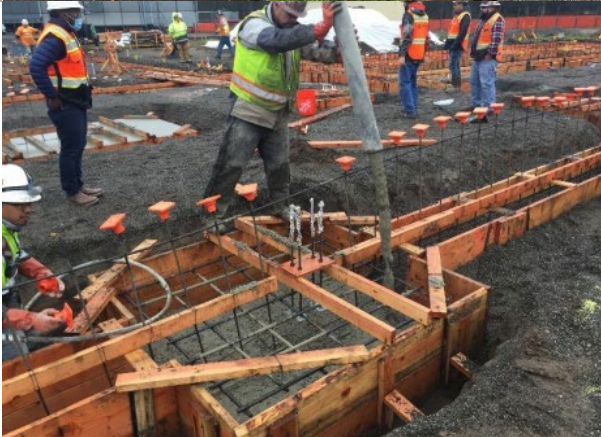
Formwork placed for foundation footings and placing concrete in a footing for a structural column.
