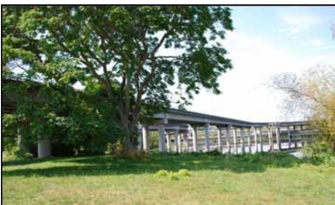
Existing view from the WSDOT peninsula looking northwest where ramps will be removed.
