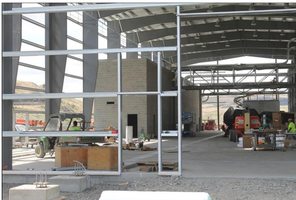
The Columbia Pulp building project has created 90 new jobs in rural Columbia County and will prevent tons of wheat straw from entering the waste stream or pollution from burning. Photo by Allan Johnson.
