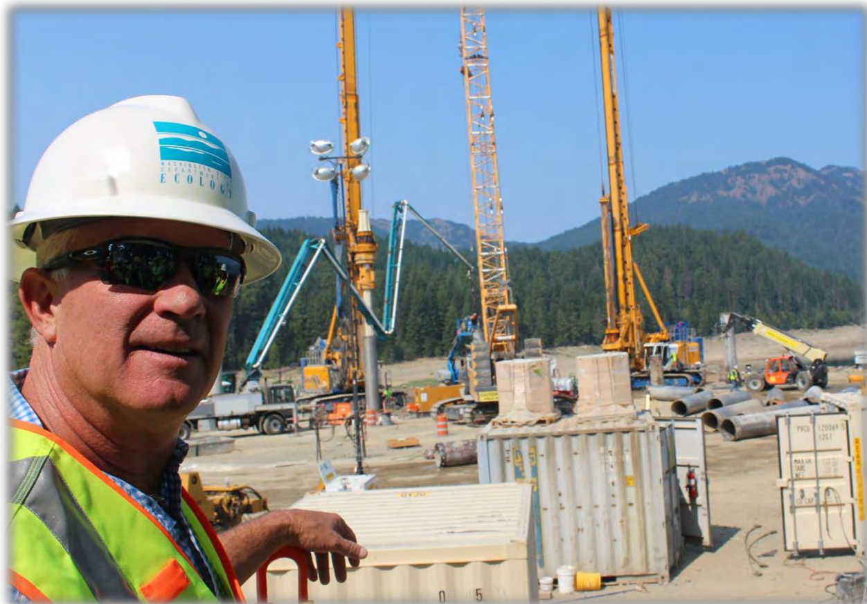
OCR's Director, Tom Tebb, at the Cle Elum Fish Passage construction site
