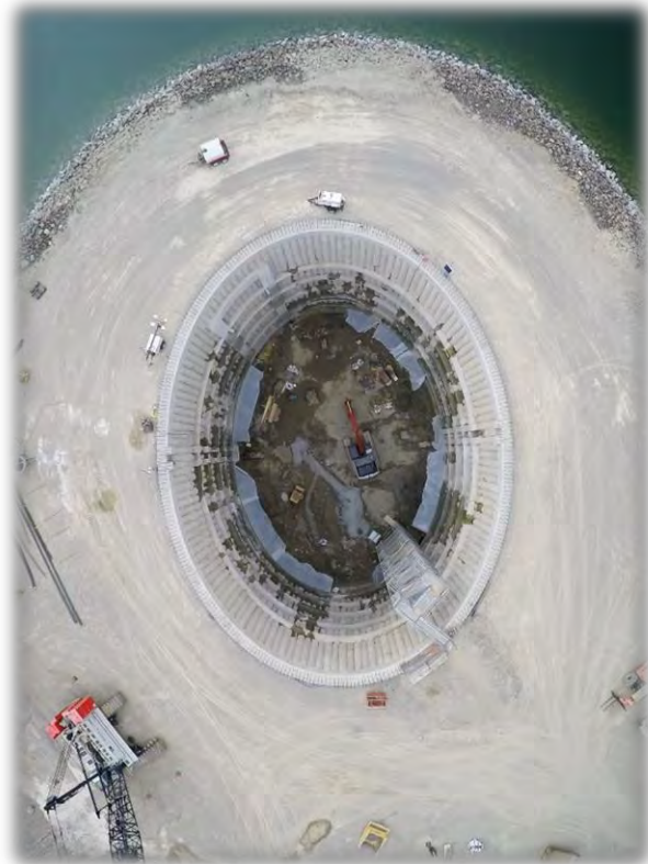
Construction of the Cle Elum juvenile passage facility vault, aerial photo provided by Reclamation
