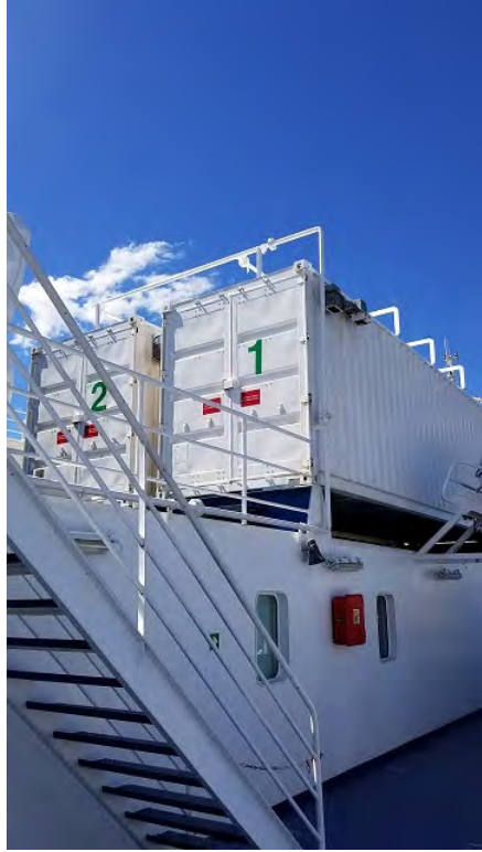
Figure 3: TYCHO BRAHE Battery Containers
