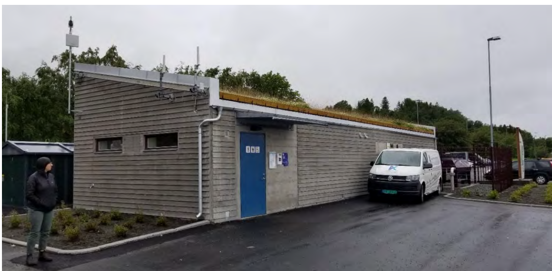
Figure 8: Shoreside Battery Bank in Flakk, Norway
