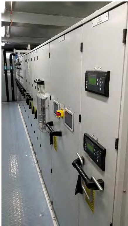
Figure 5: TYCHO BRAHE Shore Power Inverters
