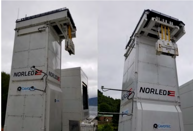
Figure 12: Cavotec APS Tower RCS
