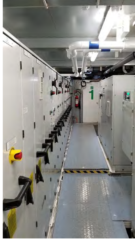
Figure 4: Interior of Converter Container
