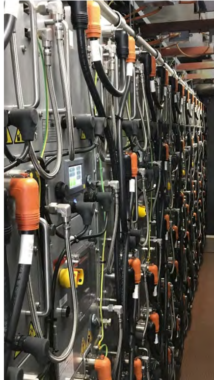
Figure 6: Sterling PBES (SPBES) Battery Racks
